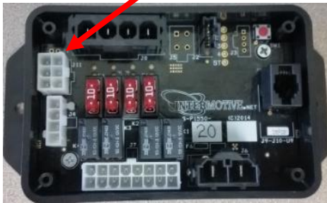
Data Link Harness plugs in here
