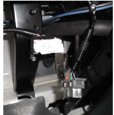
OEM OBDII bracket with White ITCEMS950 connector installed, with Grey OEM connector in lower right
